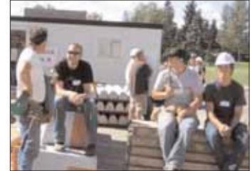
Members of West Springs Community Church in Calgary, AB build a home for Habitat for Humanity.
